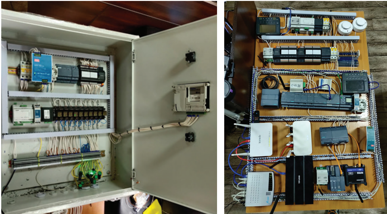
Figure 7 – Overview of the Control Box
